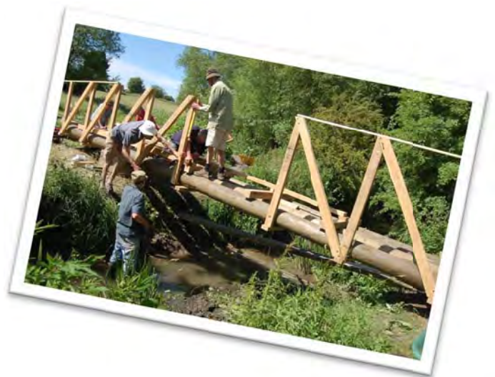
Cuttle Brook Volunteers replacing bridge at Cuttle Brook Nature Reserve in Thame (Thame Town Council)
