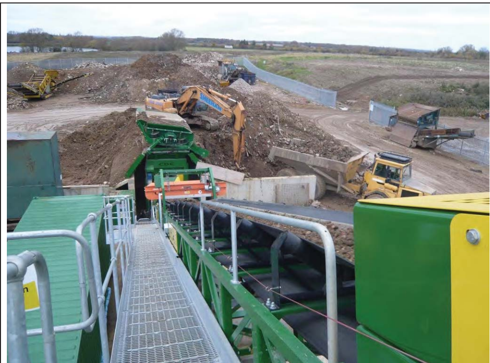
Plate 2 View of the loading of the recycled material into the plant and through the first crusher, which sorts oversized material for separate crushing. The orange box above the conveyor belt is a magnet to remove metallic constituents.
