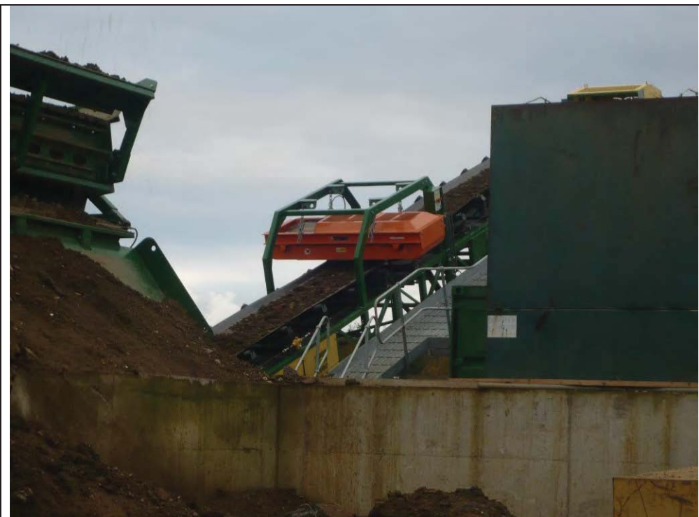
Plate 4 General view of the magnet above the conveyor belt.
